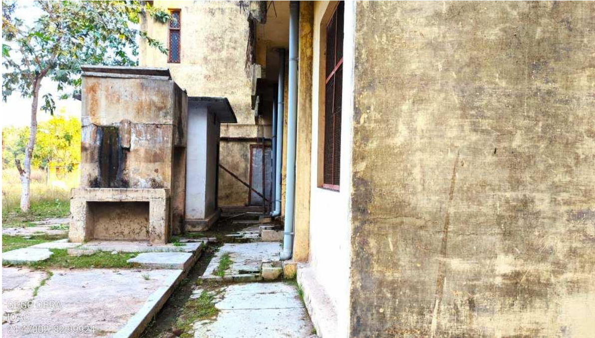
Water Drainage System from Labs
